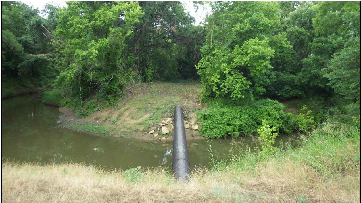
Figure 3. The existing aerial sanitary sewer across Big Bear Creek, looking southwest from the north bank.
