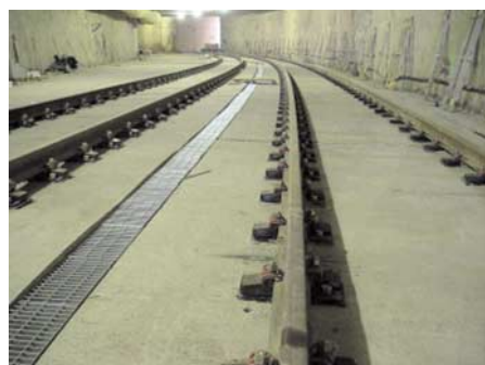
FIG. 1—Example of slab track installed in Madrid subway [1].
