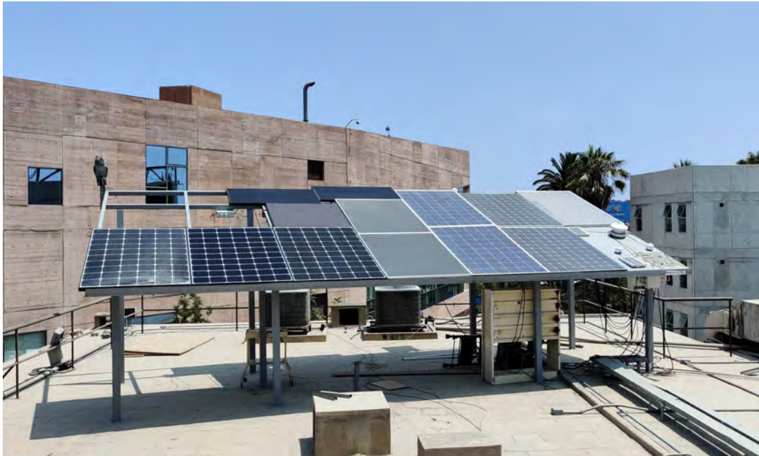
Figure 2.2: PV modules and measuring instruments installed on the roof.
