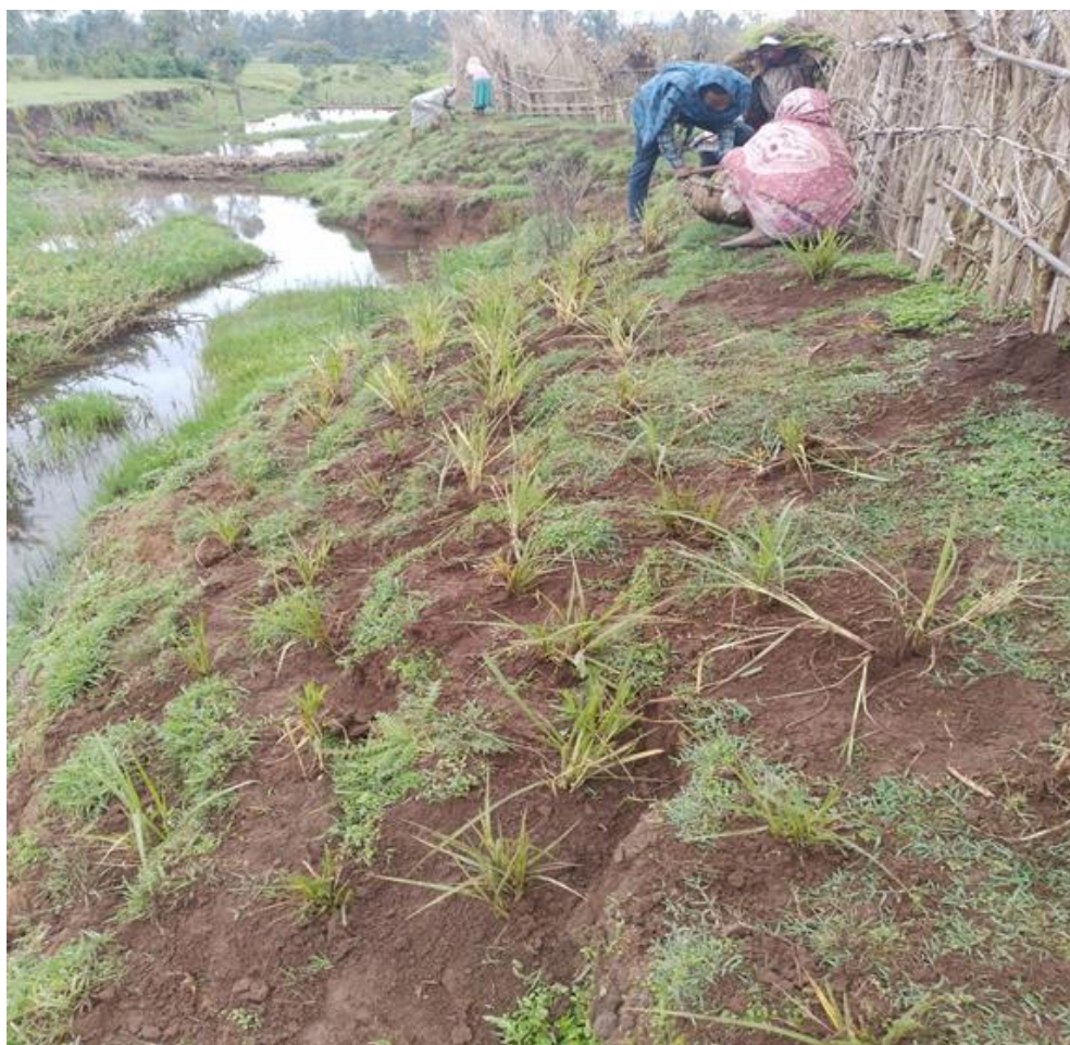
River bank stabilization and management in Amhara region, photo credit by Dessie Adane
