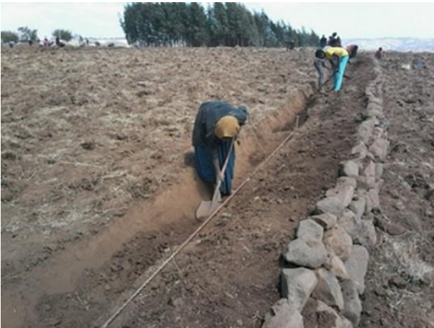
Stone faced level soil bund in Amhara region, Wogera woreda by Yaregal Fiseha
