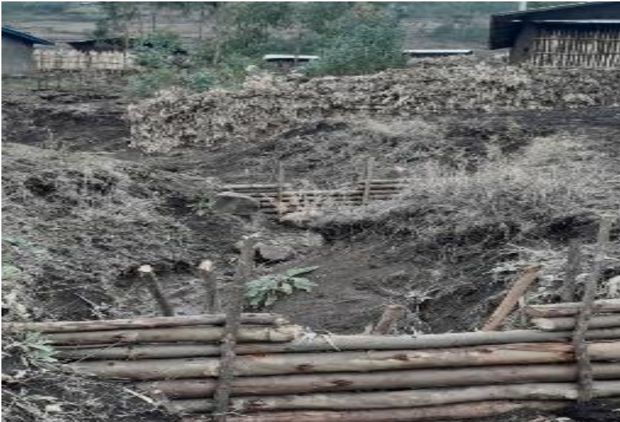
Brushwood check-dam in Bure zuriya (Amhara region), photo credit by Melisew Mengistu
