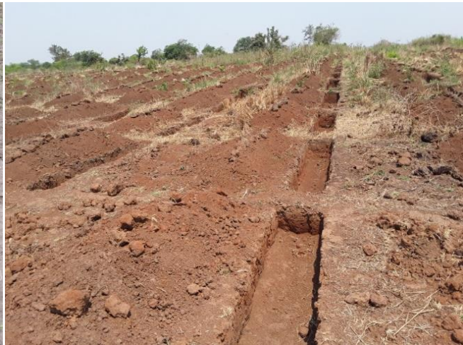
Soil faced trench in Makouy woreda, Gambella region photo by Mikre Adane
