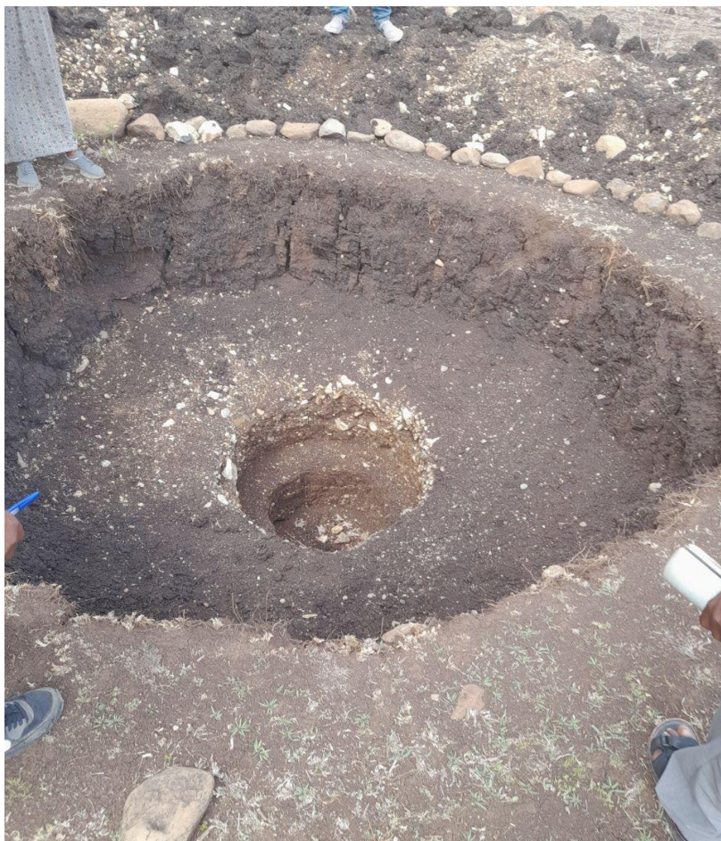
Deep percolation pit in Amhara at Takusa wored, photo credit by Angaw Zewdu
