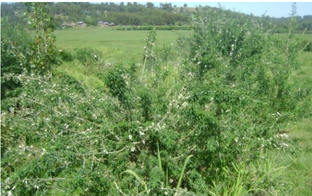
Gully stabilization using vegetation (Tree Lucerne) Dendi woreda, Oromia region, photo credit by Zenebe Adimassu
