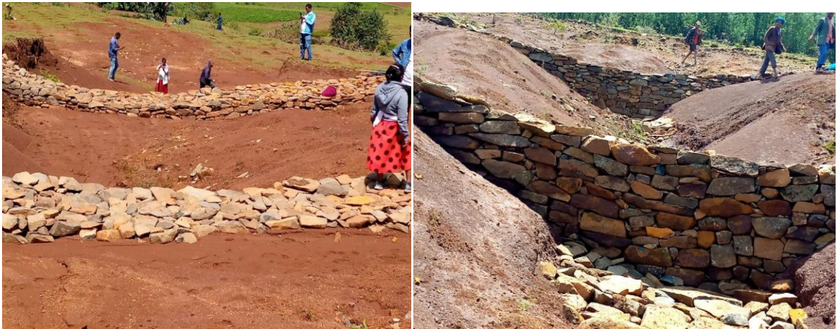
Stone wall check-dam at SeKella woreda (Amhara region), photo credit by Shibabaw Goshu
