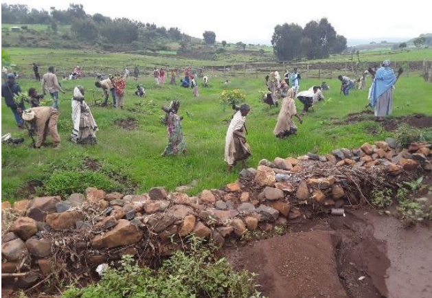
Loose rock Checkdam in Chilga woreda , Amhara region, photo credit by Daniel Tegegn
