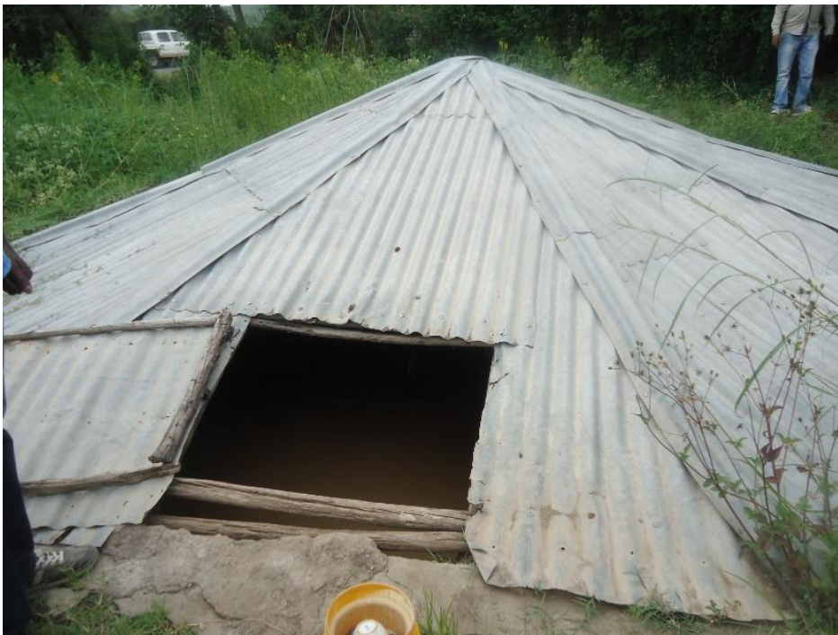
Rainwater storage tank in Adulala (Oromia region), photo credit by Abera Assefa
