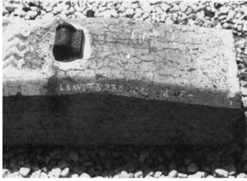
(e) delayed ettringite formation (DEF) (Hime, 1996)
