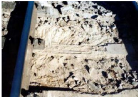
(g) bar corrosion (Mohammadzadeh and Vahabi, 2011)
