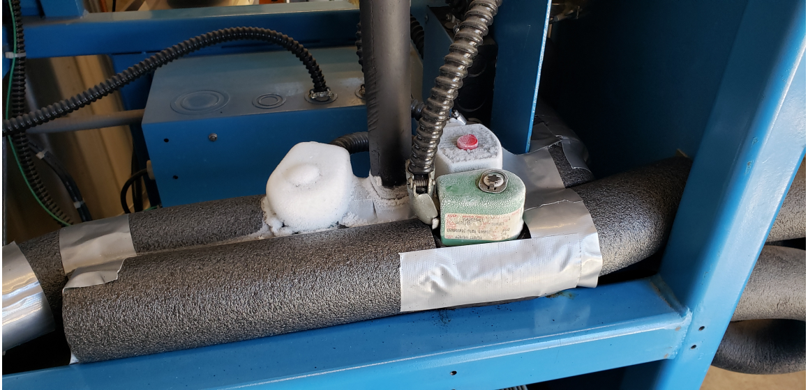
Figure 6.3: Insulation around chamber cryogenic valves and uninsulated areas with ice buildup
