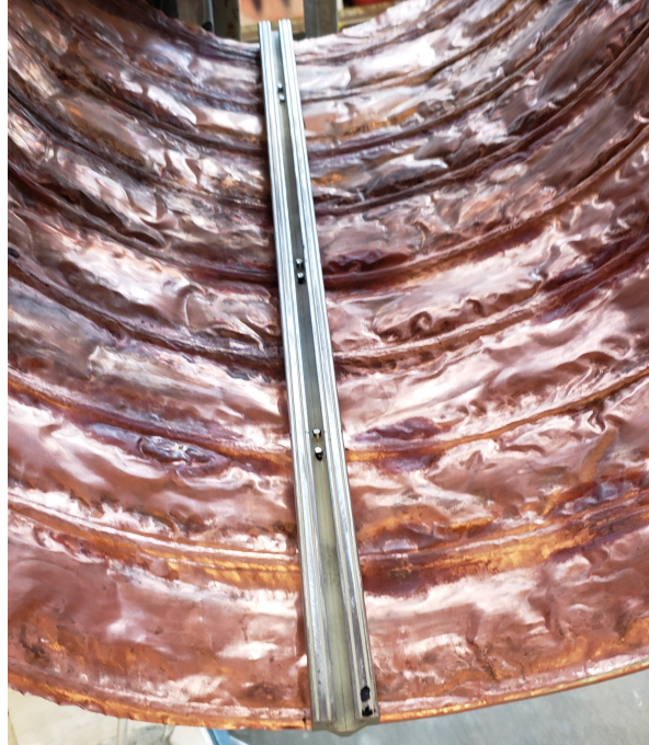
Figure 3.9: One mounting rail test fit and bolted in place to determine bolt lengths
