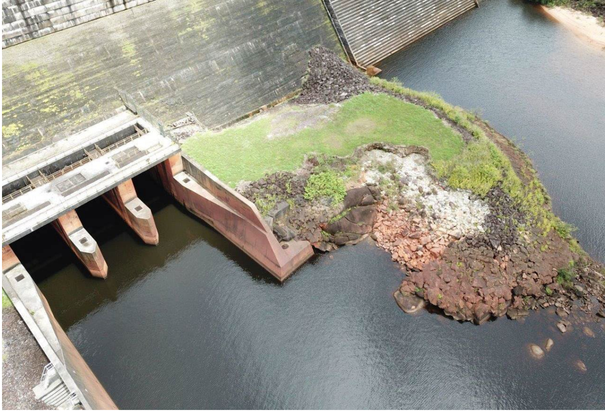
Figure 8: Erosion of the left bank to the bottom outlet (2018).
