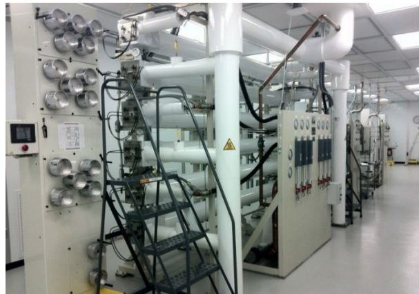
Figure A.2 Continuous stabilization and carbonization facility.
