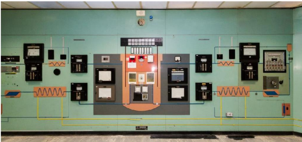
Fig. 2.9: Main DFR Control Room panel showing layout of reactor. DFR Condition Report
