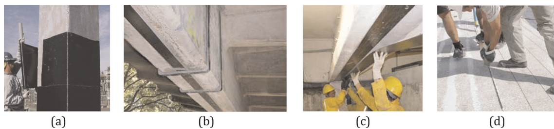
Figure 5. FRP strengthening systems [68]: (a) column strengthened with woven unidirectional carbon fibre fabric; (b) CFRP plates and strips bonded to a bridge concrete beam; (c) externally bonded CFRP plates for flexural strengthening; (d) near-surface mounted (NSM) flexural strengthening of bridge decks with CFRP rods near negative moment regions.
