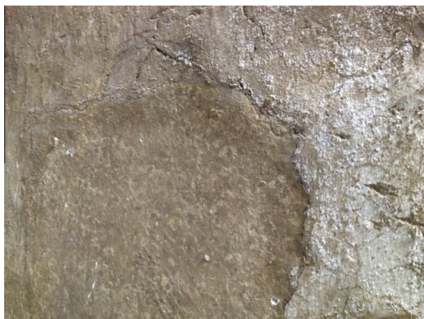
Fig. 3. Sample 1 C. Monochrome wall: white efflorescences are mainly located alongside the border of a patch composed of a different cement mix compared to the surrounding matrix.
