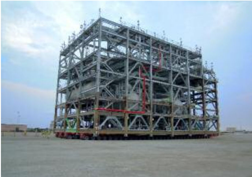
Figure 1.7 - One of the 160 modules fabricated in Thailand and then transported to Gladstone, Australia for the Queensland Curtis LNG project. Labor cost and skilled workforce availability are crucial drivers for the modularisation of the recent Australian LNG plants. (Source: Fagioli)
