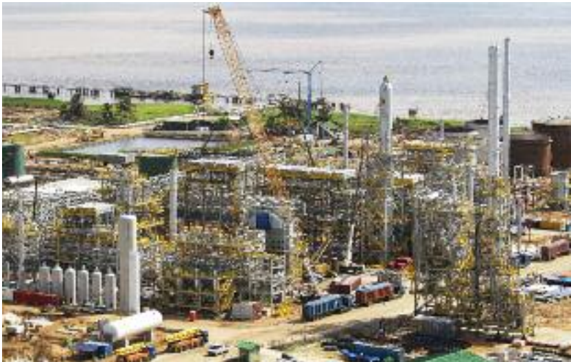
Figure 1.14 - Panoramic view of a modularized refinery performed in Suriname. An accurate analysis of the installation's sequence of the modules is a key success factor for a modularized plant's project. (Source: Saipem)
