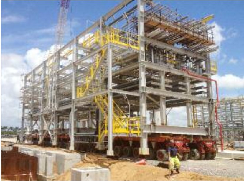
Figure 1.4 - Installation at site of a module fabricated by Saipem at Arbatax yard for a refinery in Suriname. (Source: Fagioli)
