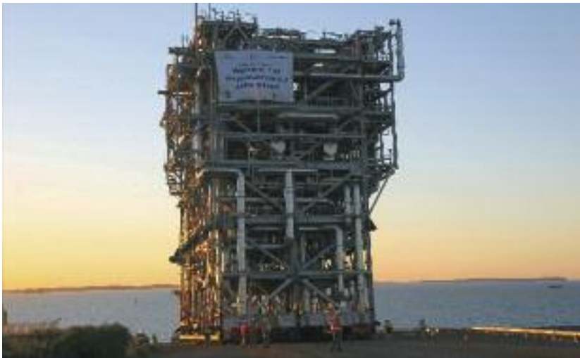
Figure 1.1 - One of the pre-assembled units for the Woodside-operated Train V Phase 5 LNG expansion facility at Karratha, Western Australia. (Source: Foster Wheeler)
