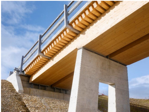
Figure 1: Bridge Horen Switzerland, block glued glulam members as main structural elements, Source: BFH, Switzerland
