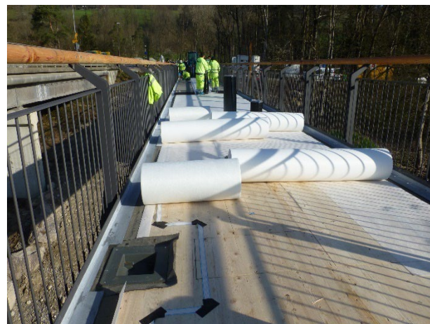
Figure 13: Sensors on the wooden panel and laying of the glass fleece and PBD seal.
