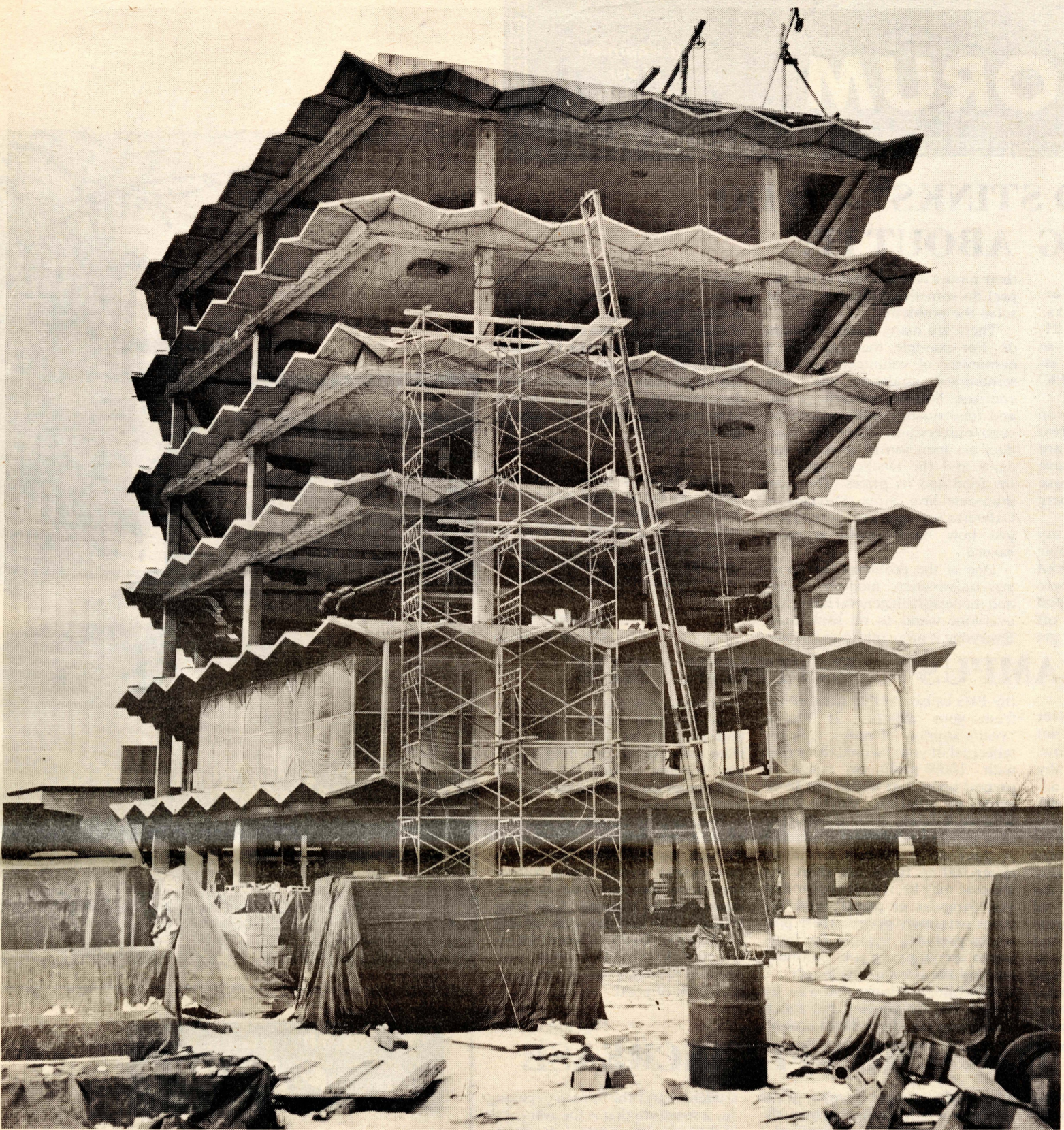
The Beehive during early stages of construction in 1960. (photo by Bill Spreitzer)
