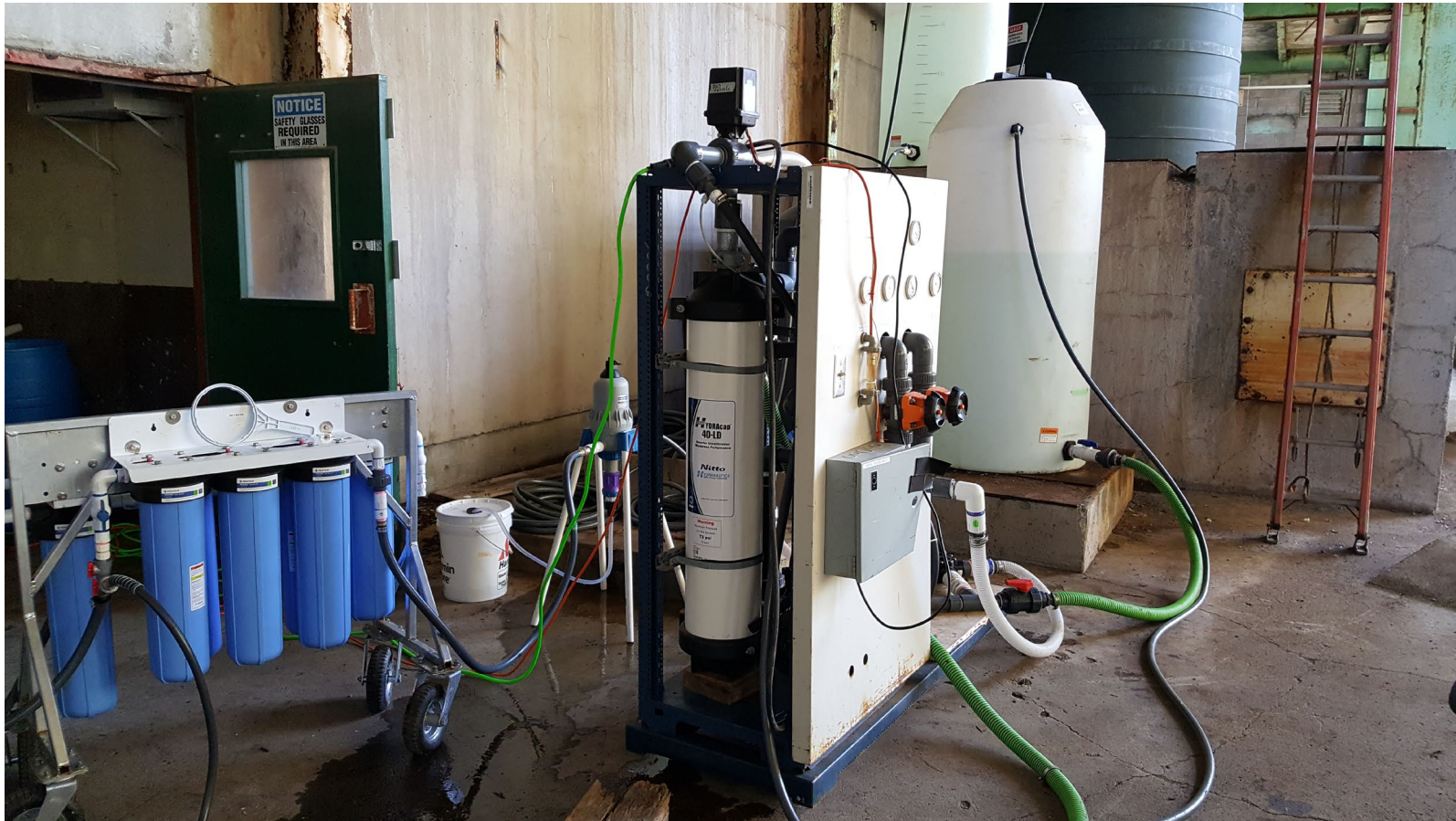
Figure 18: Pretreatment system—1. blue cartridge filters for seawater pretreatment and PRO feed carbon block treatment in lower left corner, 2. ultrafiltration unit center, 3. white seawater coagulation mix tank center right, 4. large green treated
