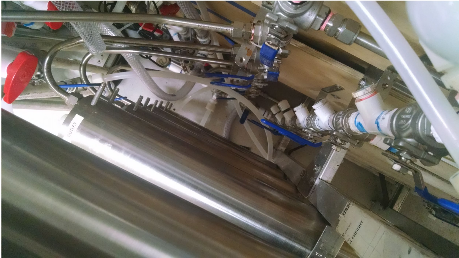
Figure 22: view of pipe network delivering feed and draw solution to PRO membrane modules. High-pressure draw solution is delivered in stainless steel tubing, and feed solution is delivered in clear plastic tubing.
