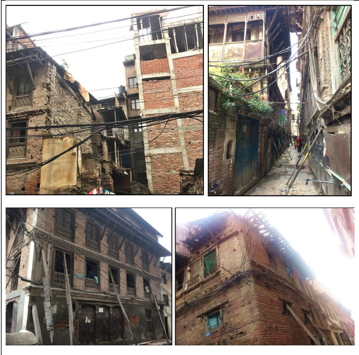
Figure 11: Damaged Private Households in Kathmandu Metropolitan City (Photos by Barsha Manandhar)
