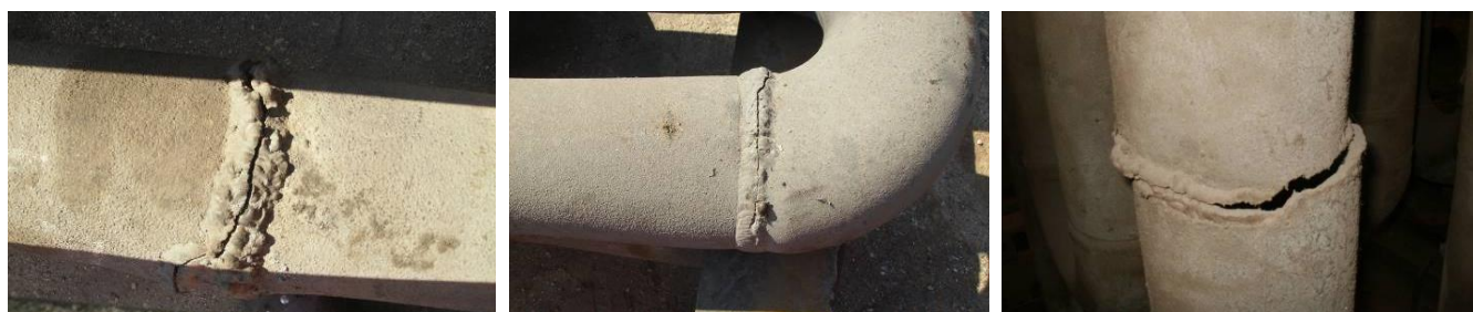
Figure 4. Cracks along the welded joint length in burner pipes.
