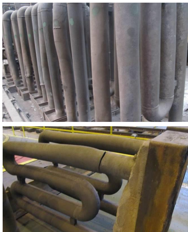
Figure 2. 'W' burner pipe input damage.
