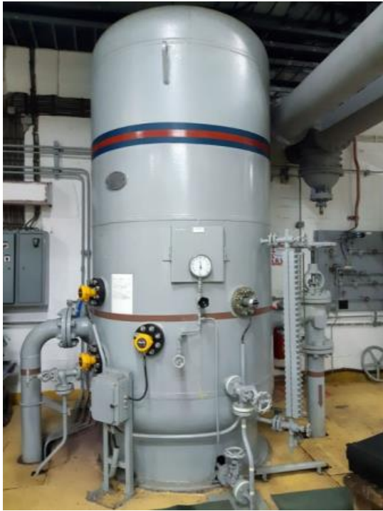
Figure 2. The pressure vessel 976 at RHEBB.
