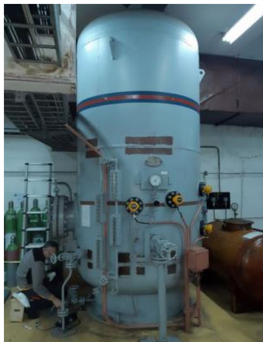
Figure 1. The pressure vessel 977 at RHEBB.
