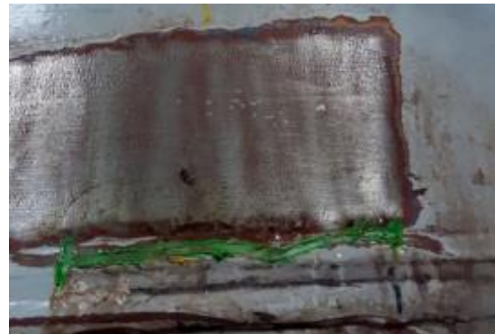
Figure 3. Position and size of defect 2.5 in vessel 977.
