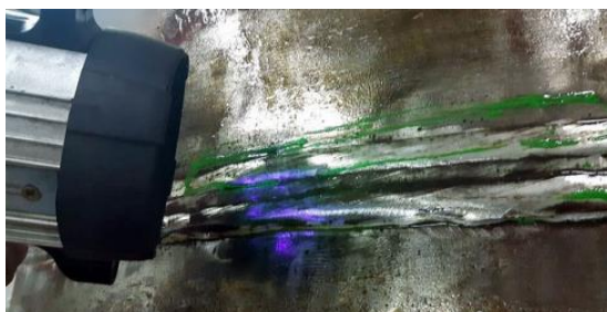
Figure 18. Magnetic particle tests on the outside wall of vessel after the repair welding of defect 2.5.
