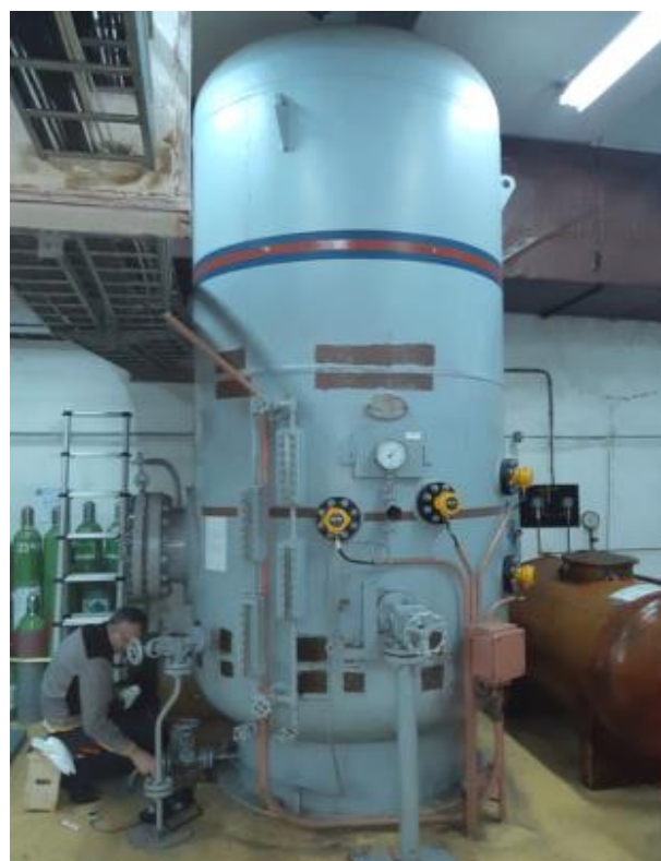
Figure 1. The pressure vessel 977 at RHE BB.
