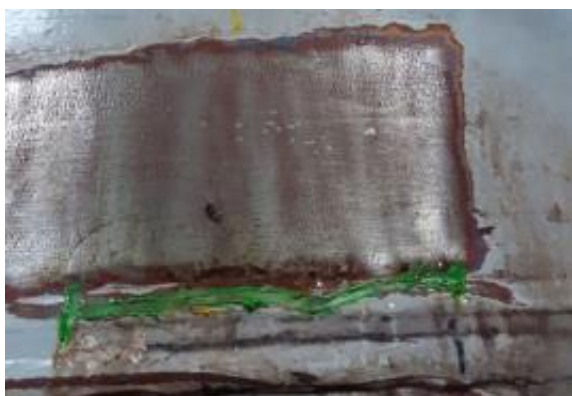
Figure 3. Position and size of defect 2.5 in vessel 977.
