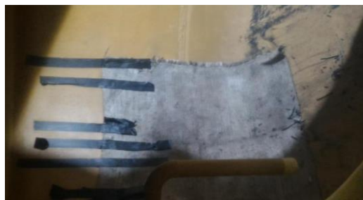
Figure 15. Asbestos cloth on the inner side of vessel.
