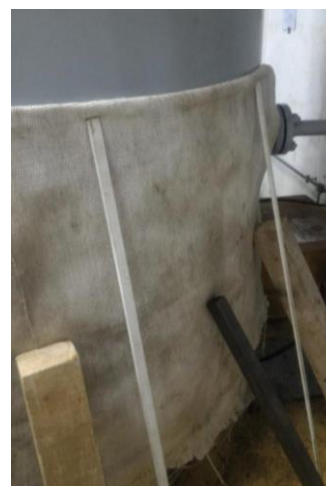
Figure 16. Asbestos cloth on the outer side of the vessel.
