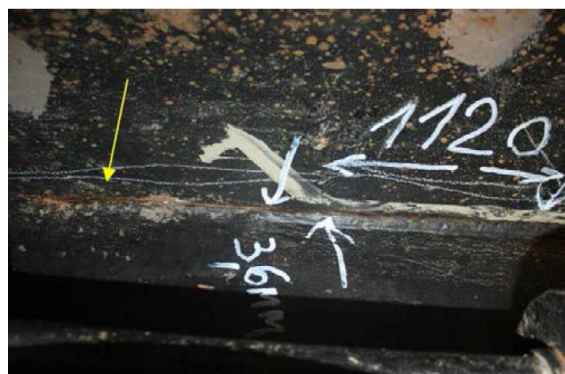
a) Crack at the welded joint of runner shield with concrete
