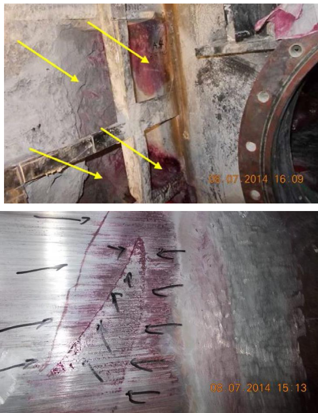
Figure 8. Characteristic surface damages in parent material and weld metal in the manhole and runner areas.
