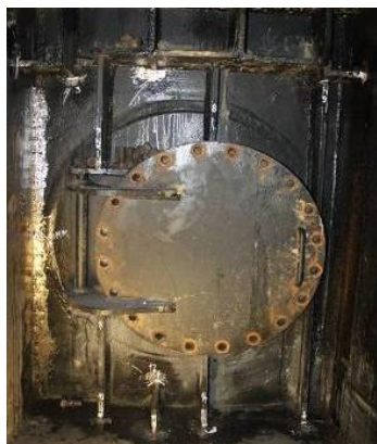
Figure 3. Kaplan turbine runner manhole as part of the hydroelectric generating set A4.
