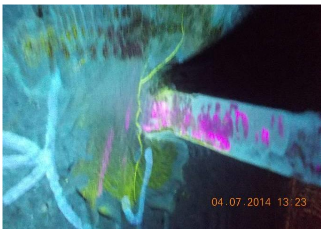
Figure 9. Surface crack detected by MT at the welded joint, between the strengthening rib and runner shield.
