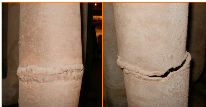
Fig. 1. Damages to the entry part of the “W” burner pipe; cracks along the welded joint.
