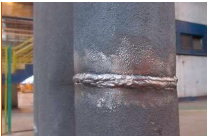
Fig. 4. The appearance of the repaired burner pipe.
