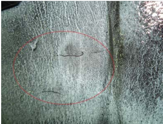
Figure 2. Crack detected by MT.
