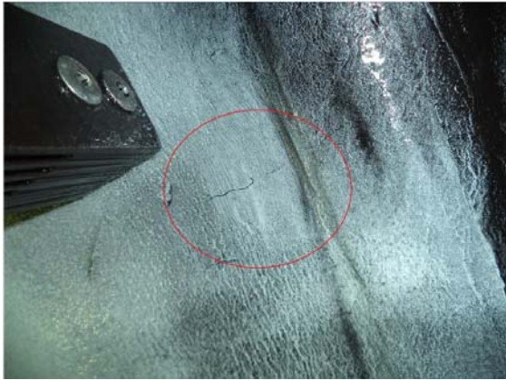
Figure 1. Crack detected by MT.
