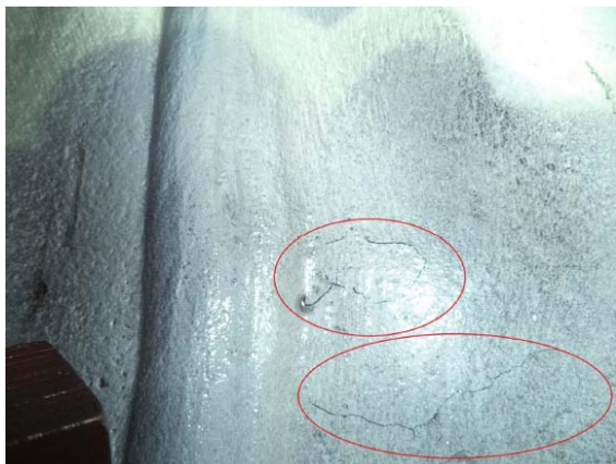
Figure 4. Crack detected by MT.
