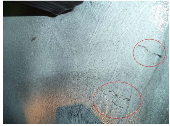
Figure 8. Crack detected by MT.
