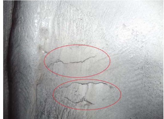
Figure 5. Crack detected by MT.
