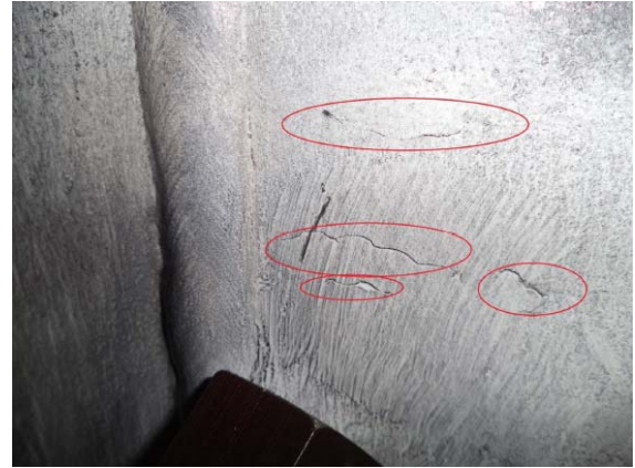
Figure 7. Crack detected by MT.
