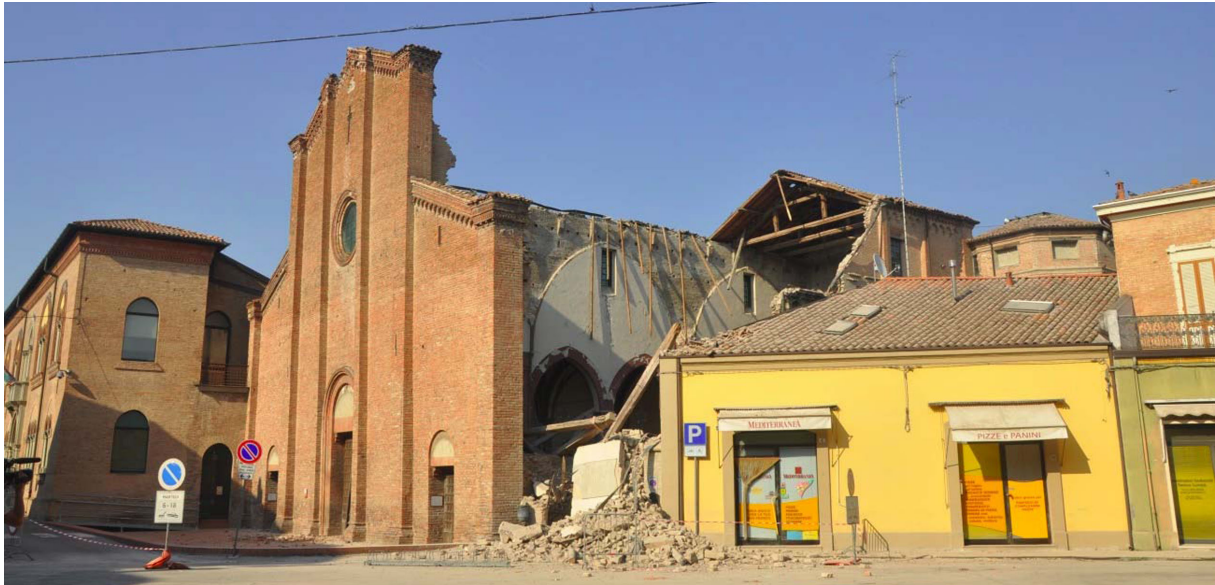
Figure 7. Collapse of the San Francesco Church (XV century), Mirandola. Courtesy of A. Penna.
