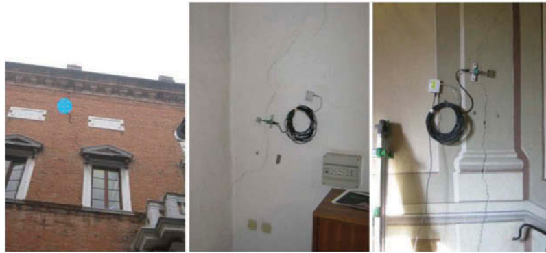
FIG. 9. Photographs showing the orientation of the cracks and position of the sensors in Figure 8: sensor A (left), sensor B (center), sensor C (right).
