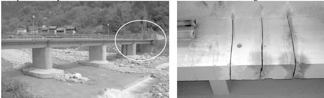
Figure 1. General view of Dogna Bridge (left) and detail of damages D1-D6 (right).
