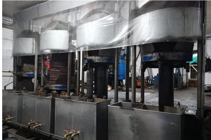
Figure 9. Decantation tanks used in the traditional mill.
