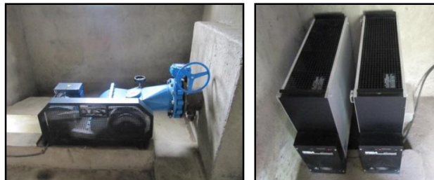
Fig. 9 Banki turbine and generator – Dump loads
