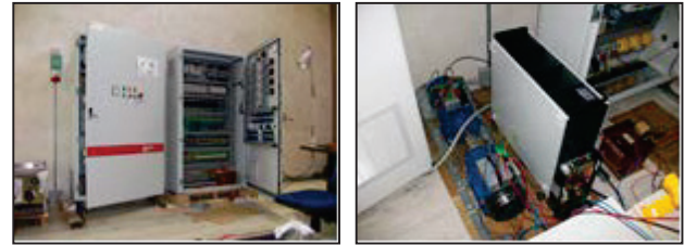
Fig. 13. Q1 and Q2 switchboards – DC motor and ELC dump loads
