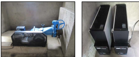
Fig. 2 Banki turbine and generator – Dump loads
