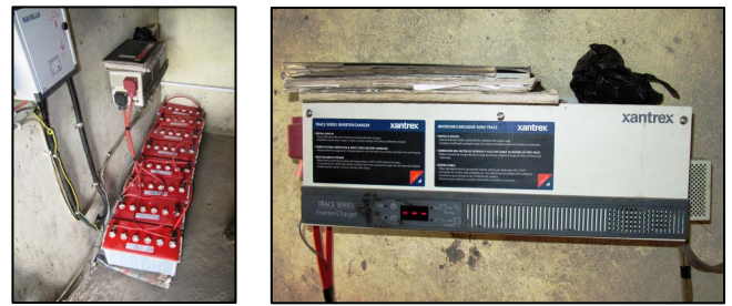
Fig. 3 Battery pack and charge inverter coupled with the AC system
