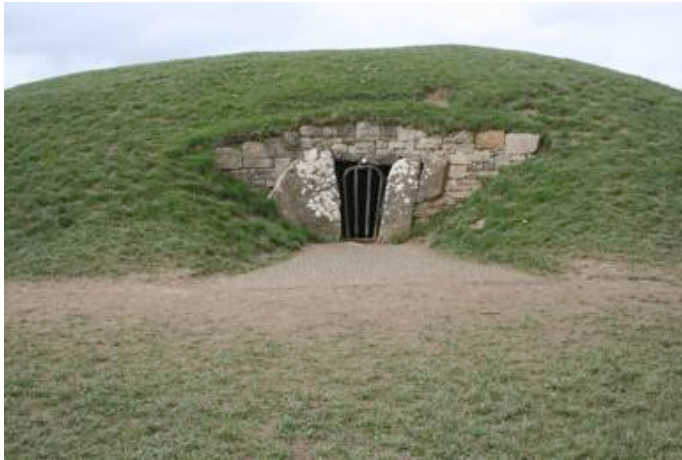
Fig. 15 East-facing entrance to the passage tomb, showing turf reinforcement mesh extending from entrance to edge of mound and extensive erosion from pedestrian traffic (April 2018).
