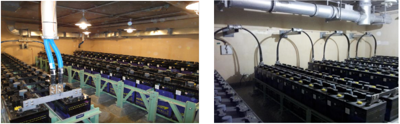
Figure 3: Two separate battery rooms in nuclear power plants [17, 18].
