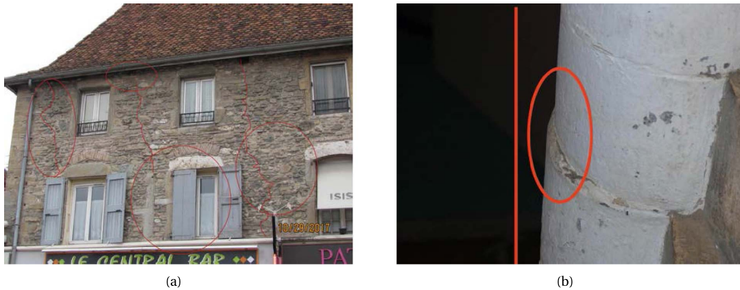
Figure 5. (a) House in the town of La Tour du Pin, reconstructions marked in the red circles, filled cracks indicated by the red lines, an opening reduced in central part of the wall, and a reconstruction with small bricks at the upper part between the two windows. (b) The “Dolphin House” (16th century) at La Tour du Pin, the stair’s barrel broken and shifted, with the loss of vertical alignment as shown by the red line [Poursoulis, 2017].
