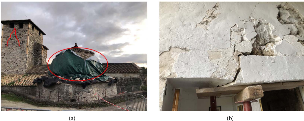
Figure 8. (a) Saint-Etienne of Melas church (assumed construction date: 11th century): degradation of the cover of the baptistry in the red ellipsoid, cracks in the bell tower indicated by the red lines. (b) Castel of Saint-Tomé (assumed construction date: 14th century), broken lintel.
