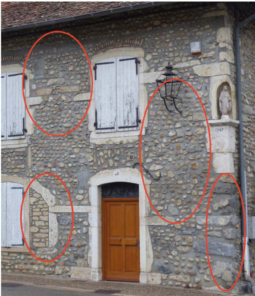
Figure 6. Damages and repairs observed for a masonry house (extracted from Poursoulis [2017]).
