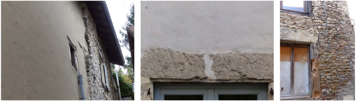
Figure 5. Examples of traces of damage in masonry structures: peeling of a wall, broken lintel, and crack in a wall (extracted from Poursoulis [2017]).
