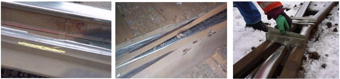
Figure 12. The worn switch rail, where the crack had formed from the railhead down to the metal, propagated longitudinally and gradually turned upwards again, causing a large part of the switch rail to be removed (A), Spalling (loss of material chips) on a manganese crossing nose (B), the nose is worn as shown by the vertical distance between the template and the nose (C) [21].
