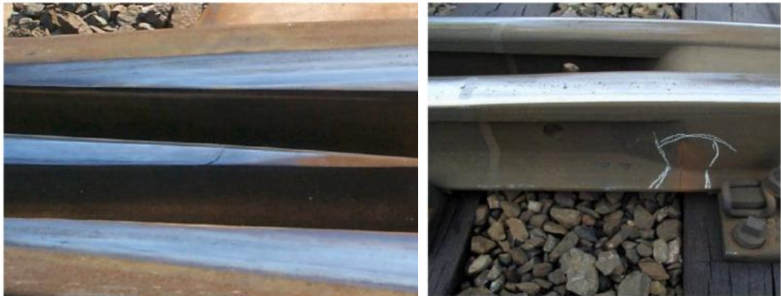
Figure 24. Cracks running transversely over the crossing nose (left), Cracks running transversely over the crossing foot (right) [32].
