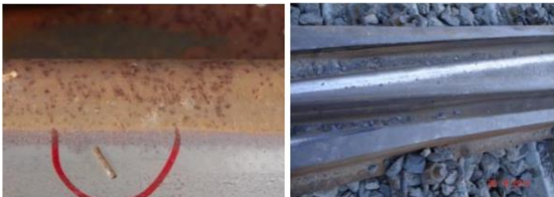
Figure 22. Showing imprints defects [158].
