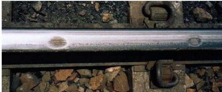
Figure 21. Showing multiple wheel burn defects [30].
