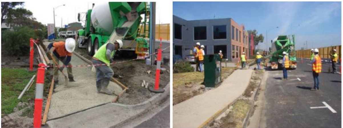
Figure 2.3 - In-situ production of E-Crete footpaths at Brady St in Port Melbourne, Australia [122].
