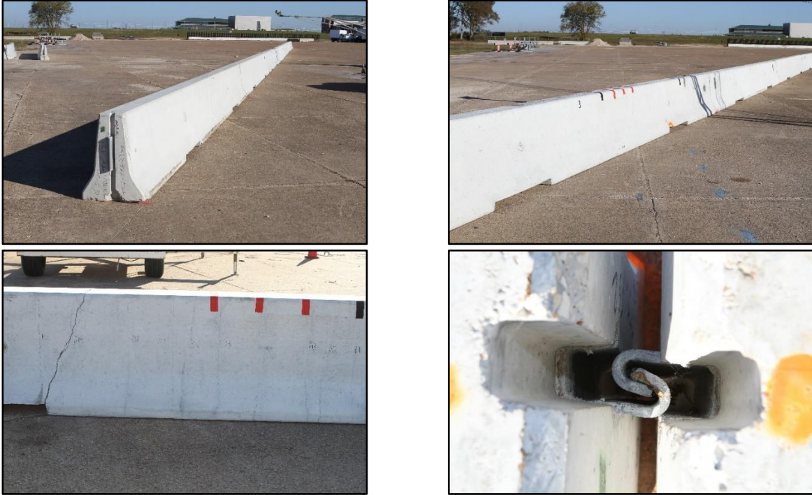
Figure 8.1. Damaged Portable Concrete Barrier before Test No. 440592-1.
