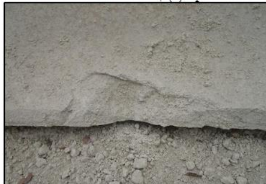
a. Spall on the Middle Base of the Barrier
