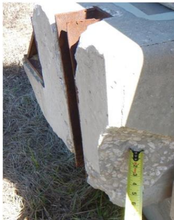
Figure 2.20. Example of Unacceptable Barrier— FDOT (31) .
