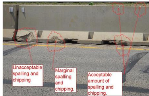
Figure 3.4. Spalling and Chipping—WisDOT (43).
