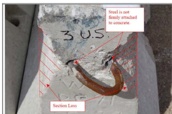
Figure 3.6. Loop Unacceptable Condition—WisDOT (43).
