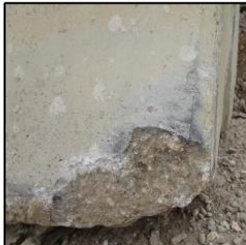
b. Spall on the Toe of the Barrier
