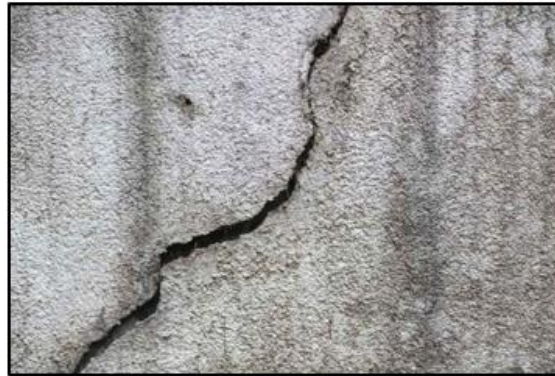
Figure 2.8. Crack Due to the Formation of More Voluminous Products (20).
