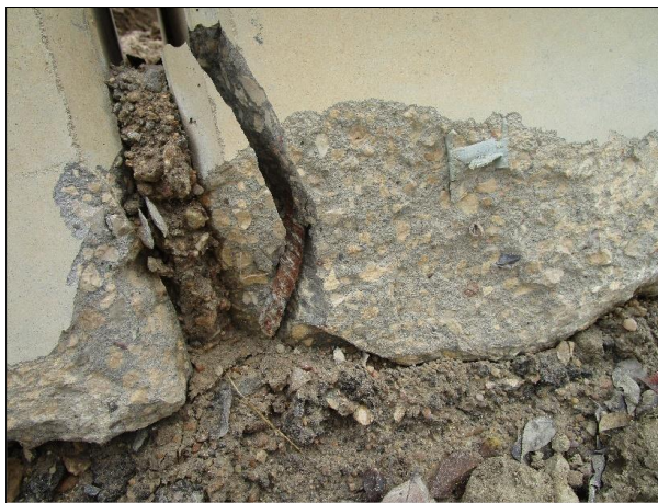
Figure 2.2. Corrosion of Reinforcing Bar Embedded in the Toe of the Concrete Barrier.
