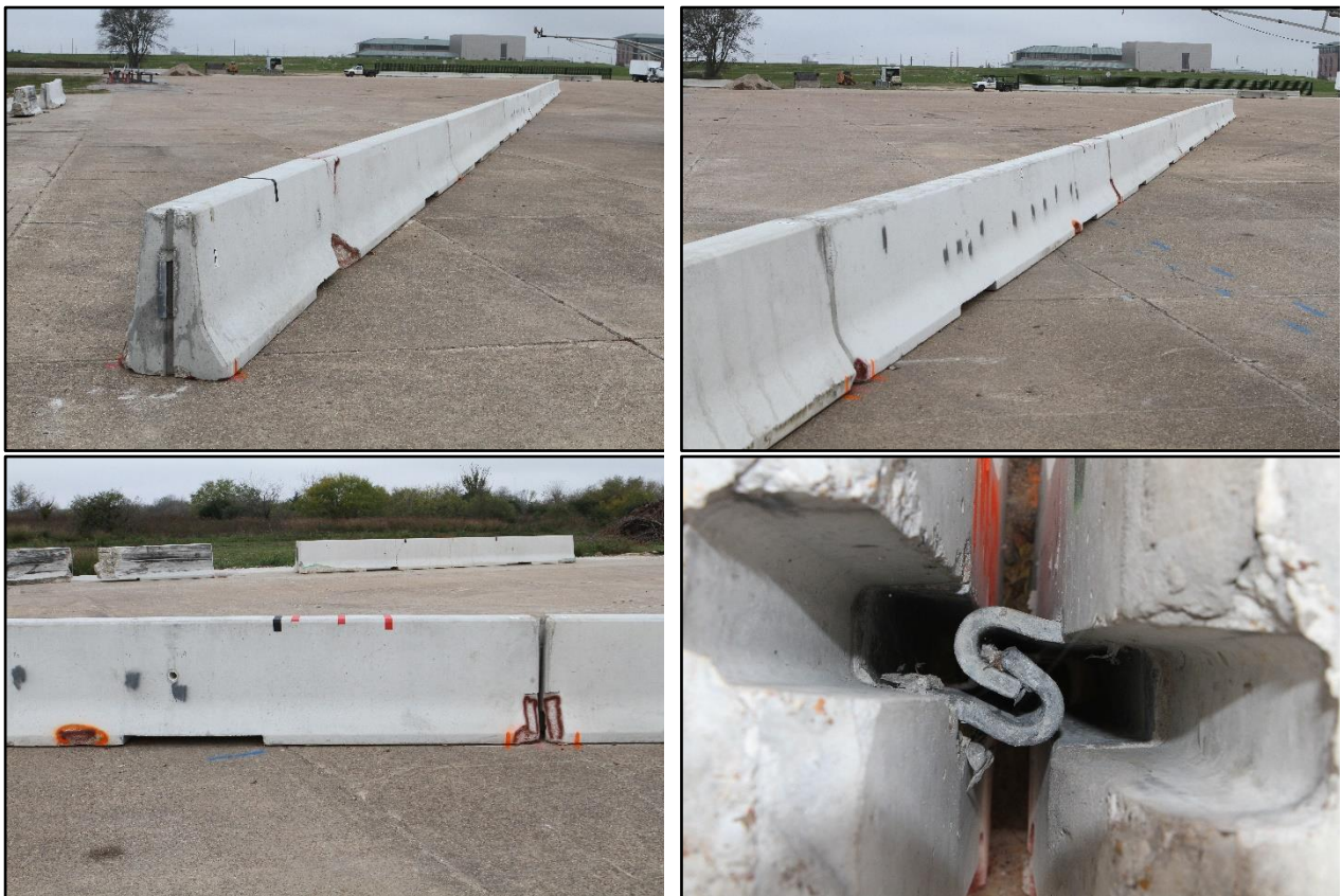
Figure 8.2. Damaged Portable Concrete Barrier before Test No. 440592-2.
