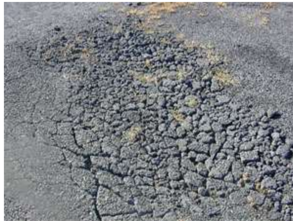
Figure 5 Alligator cracking in AC surface
