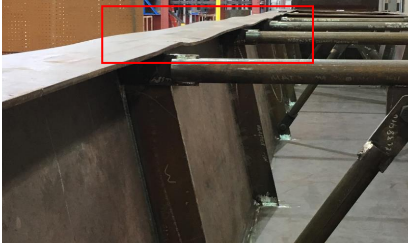
Figure 4-13 Baseline Specimen with Significant Plate Waviness on the Top Flanges
