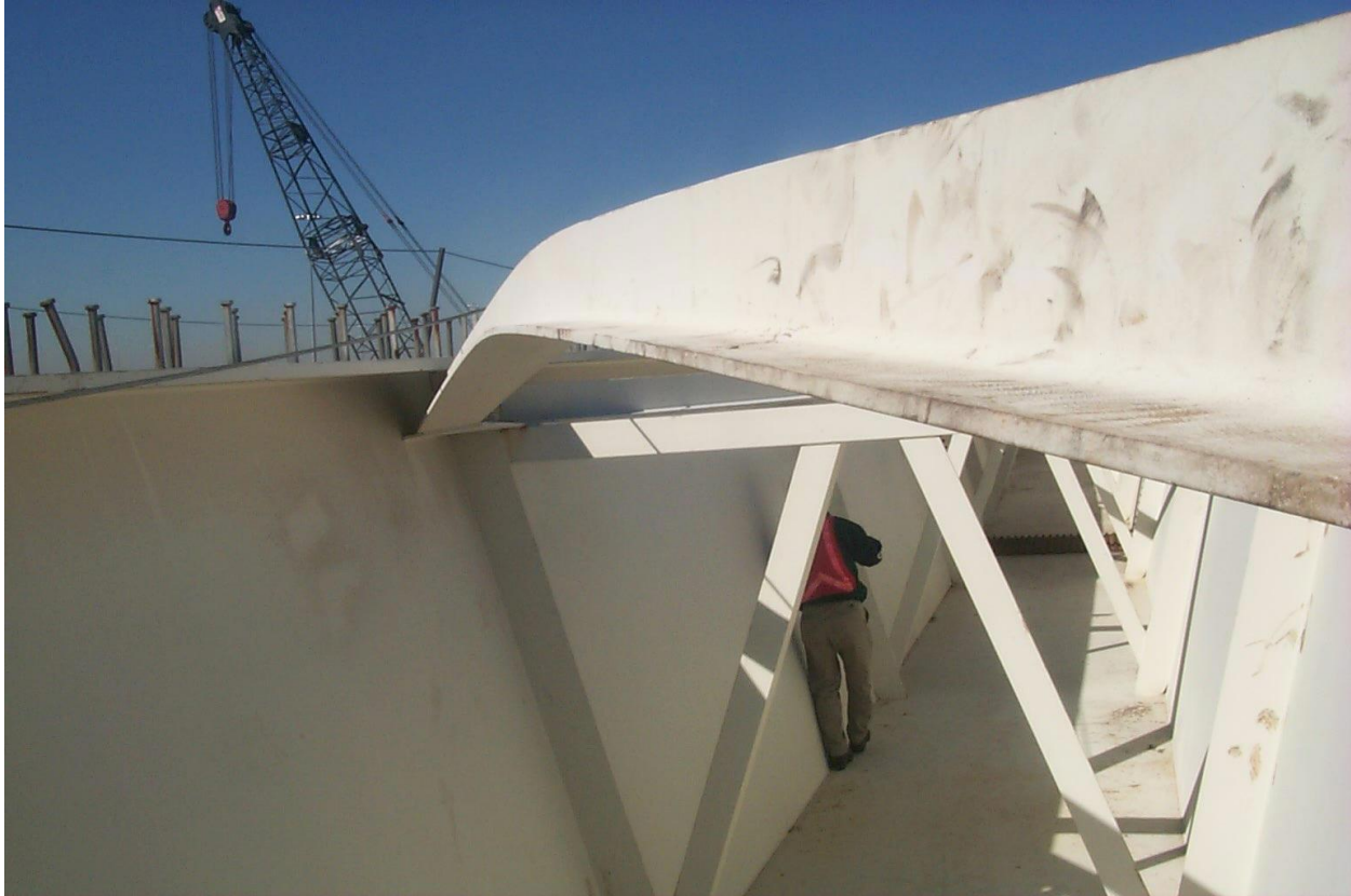
Figure 2-8 Buckling of Diagonals in Top Lateral Truss of Steel Tub Girder
