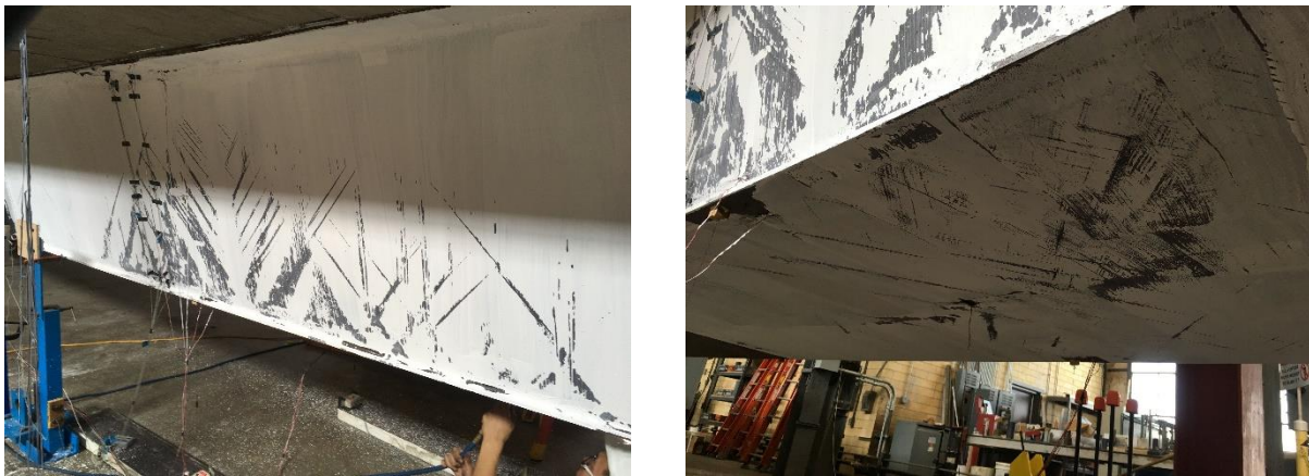
Figure 5-29 - White Wash Showing Yielding: West Web (left), and Bottom Flange (right)
