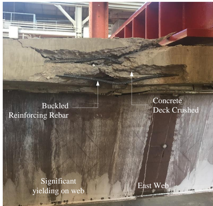
Figure 5-39 - Concrete Deck Crushed and Top Web Buckled – Tub #3
