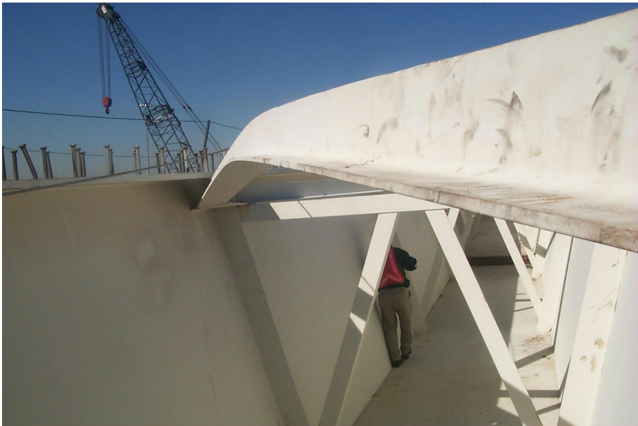
Figure 1-4 -Improperly Sized Top Lateral Truss Resulted in Buckled Diagonal
