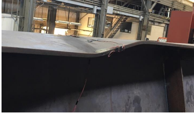
Figure 3-55 - Local Buckling of West Top Flange of Tub #2 at Midspan – View 1
