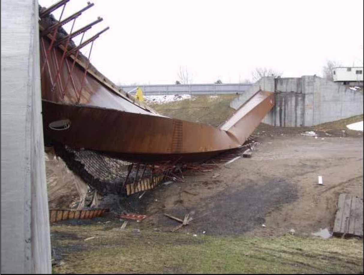
Figure 2-7- Collapse of Marcy Pedestrian Bridge (Structure Magazine, February 2008)
