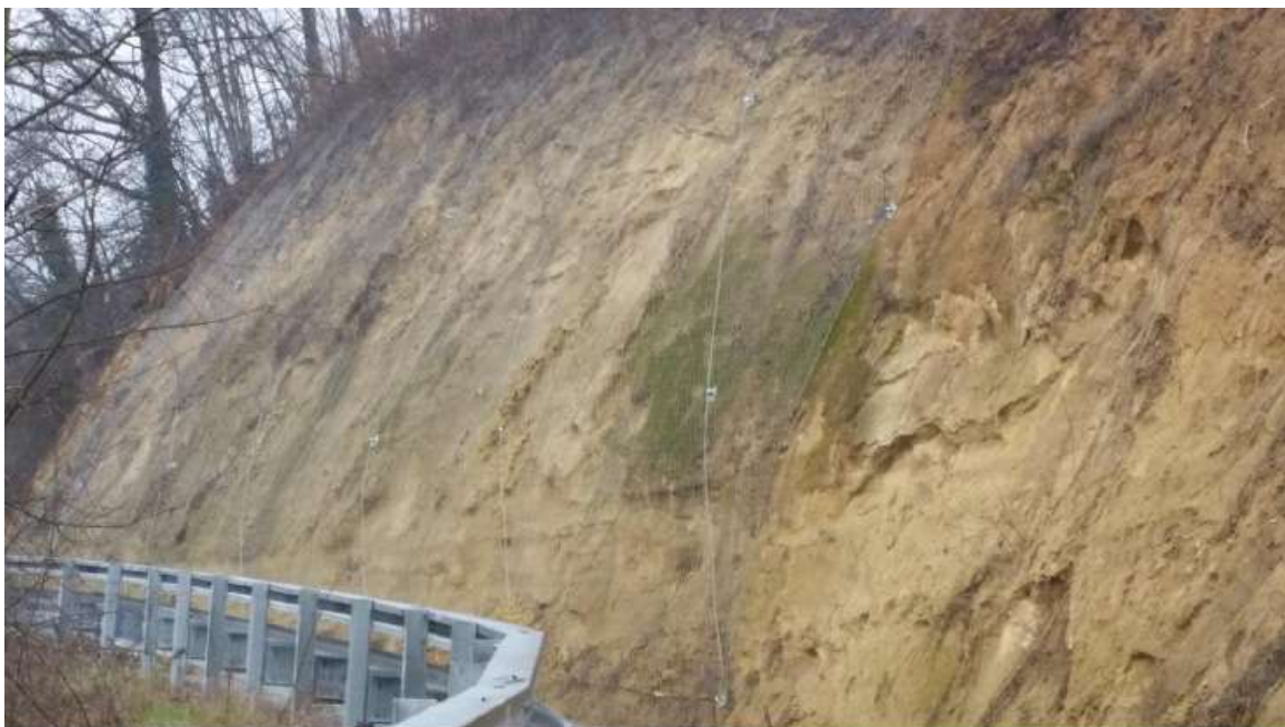
Figure 1. Metal mesh containment adhering to the Sabbie di Asti outcrops to mitigate the risk of falls on the viability.
