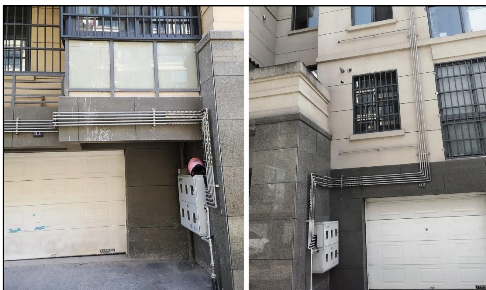
Figure 7.13. The newly-introduced gas pipes had to be installed outside the buildings (source: Author).
