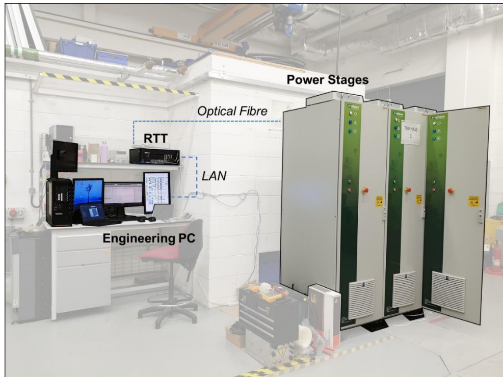
Fig 5-6 Triphase power-HIL simulator rig and associated equipment and computers
