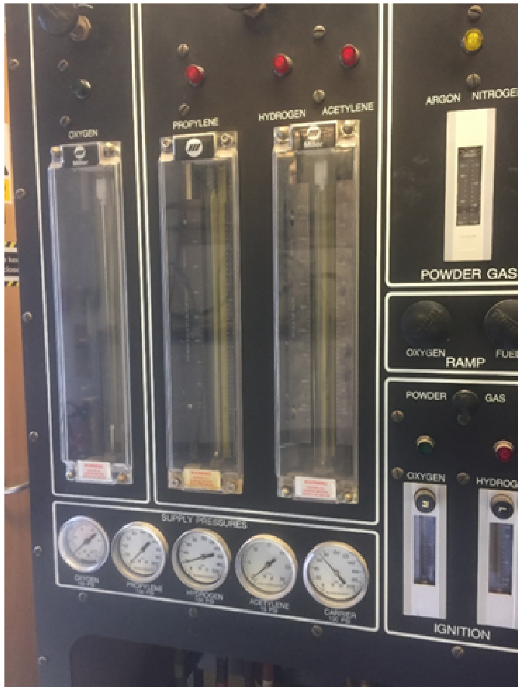
Figure 3.3: Gas flow meter control unit.
