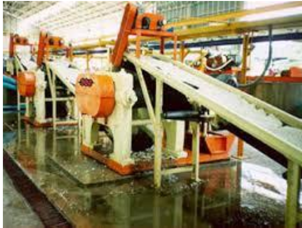
Figure 1.6: Belt conveyor system to transfer rubber
