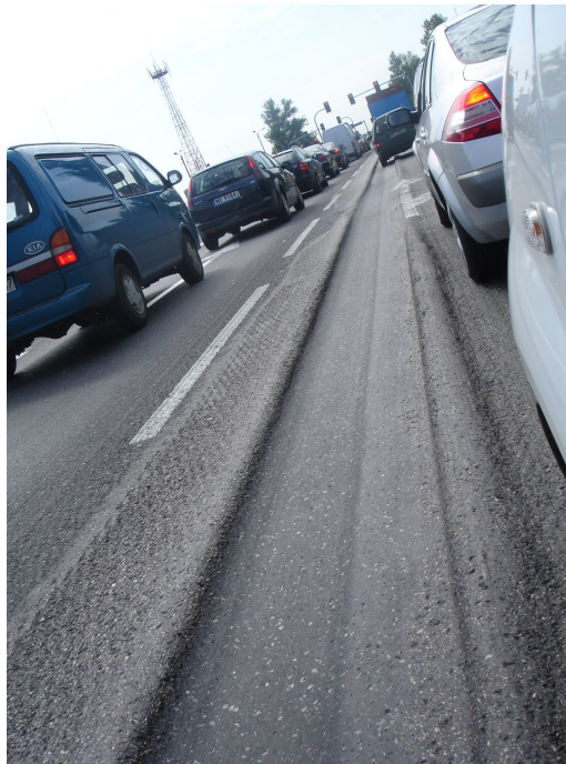
Figure 1.4: Rutting in road pavements [Google Images]
