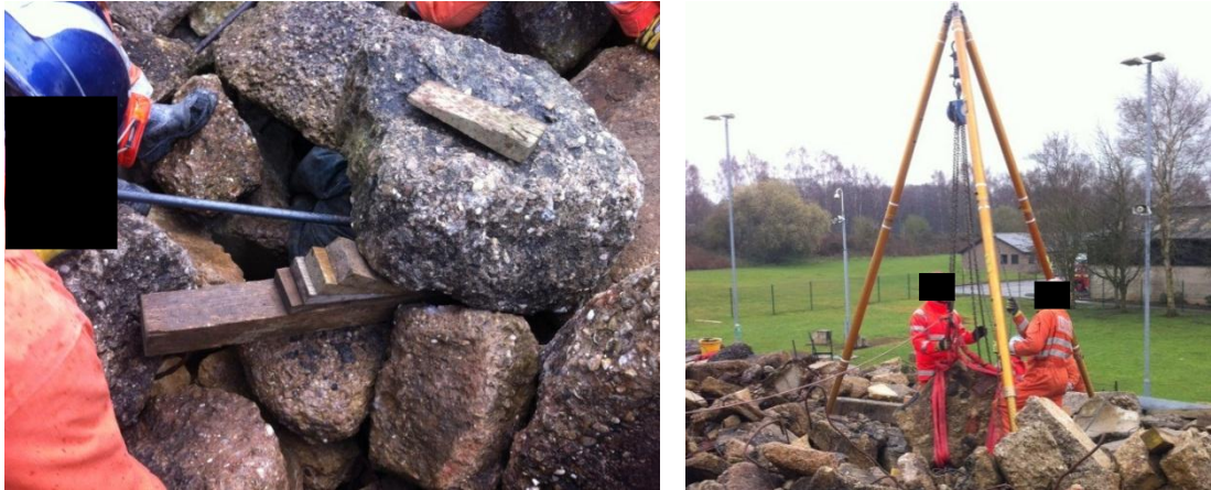
Figure 52 - Casualty extrication with crow bars and wedges (left) and Paratech tripod for lifting (right)
