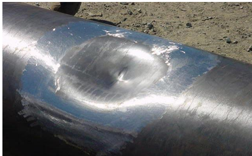
Figure 2-1, Mechanical gouge dent on a pipe
