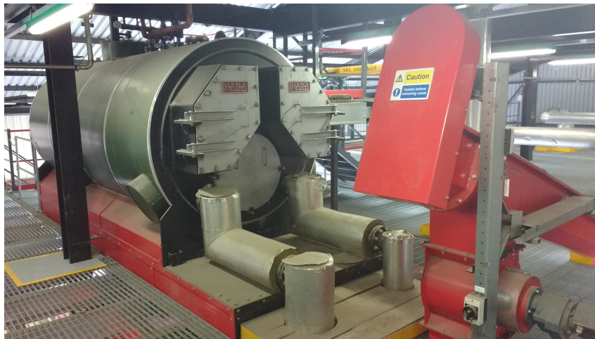
Figure A.3: Byker heat station Thermax boilers
