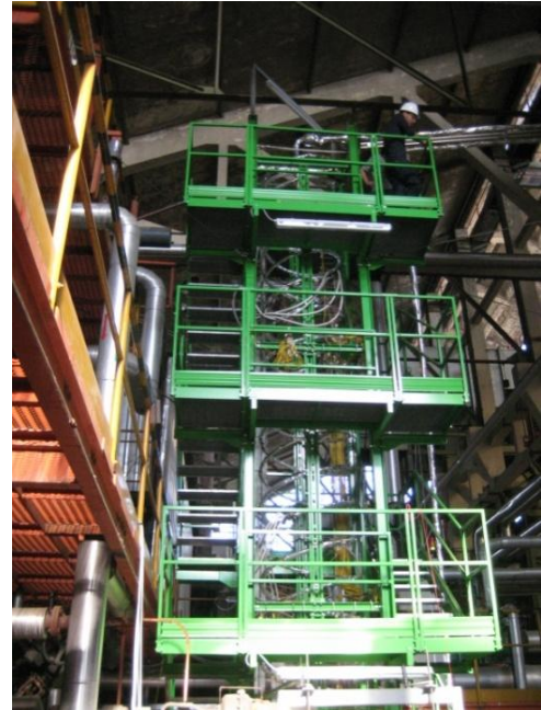
Fig. 2. Global view of the facility test section.
