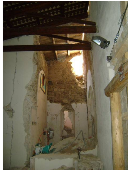
Figure 13: the collapse of the masonry wall behind the lateral chapel.
