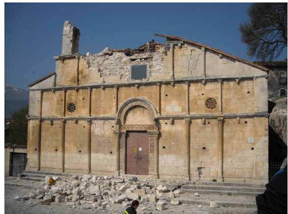
Figure 2: The façade of St. Giusta church after the earthquake of 06.04.2009.
