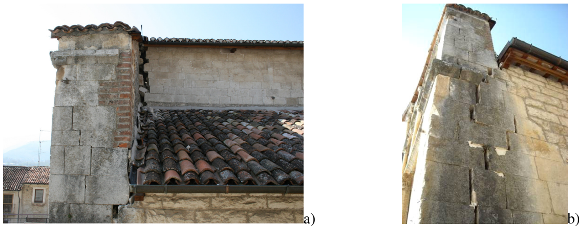
Figure 10: Detachment of the longitudinal masonry walls from the façade: a) higher part and b) lower part.
